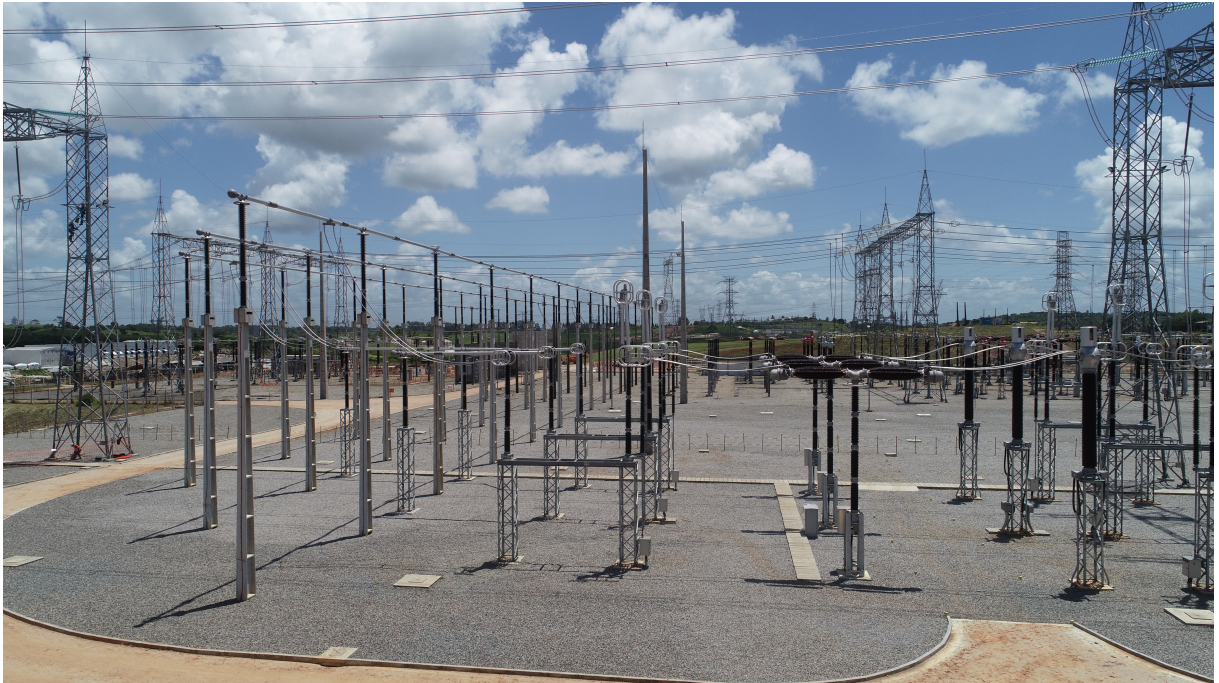
Figure 4.17: Photograph close to the HV insulators of the “UTE Porto de Sergipe I” substation.
